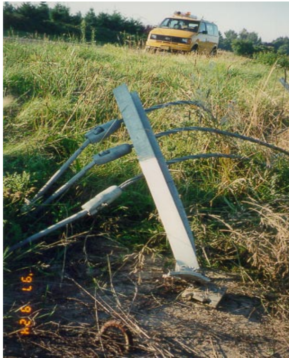
Figure 3.8: Energy dissipation-cable release from breakaway anchor angle and anchor post slip base failure
