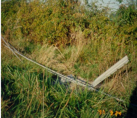
Figure 3.6: Energy dissipation-cable release from breakaway anchor angle and anchor post bracket (south end)
