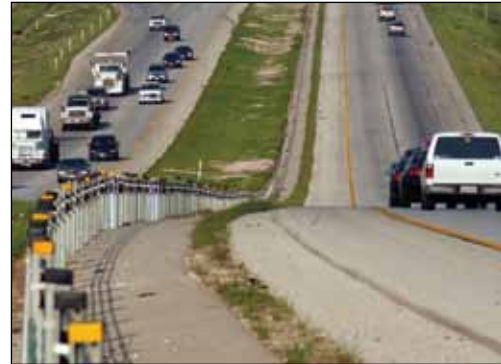
This CMB installed along IH 20 in Texas had an immediate impact in reducing the number of fatalities from cross median collisions.
