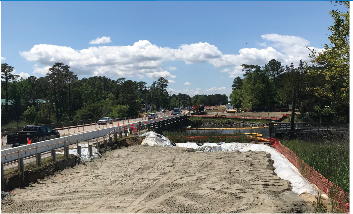
▶ This photograph shows construction work starting on the Laskin Road Bridge Replacement & Widening Project as this project was awarded in Fall 2019.
