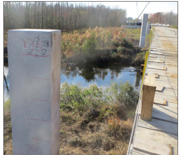
Corrosion-free CFRP piles adjacent to West Neck Creek after restrike and redrive, with a final elevation of 61'.
