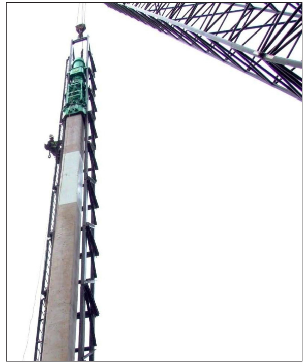
Pre-stressed pile with corrosion-free CFRP reinforcement being driven at the Nimmo Parkway Bridge site in Virginia Beach, Virginia.
