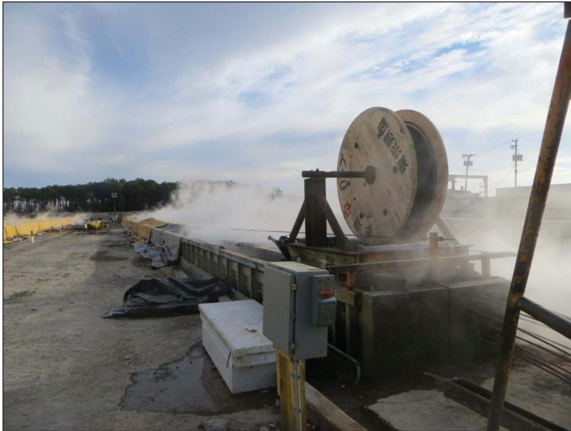
CFRP piles being steam-cured after stressing of the strands and concrete placement. A spool of CFRP strand can be seen above the stressing bed.
