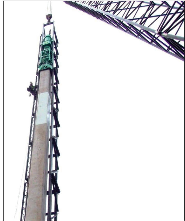
Pre-stressed pile with corrosion-free CFRP reinforcement being driven at the Nimmo Parkway Bridge site in Virginia Beach, Virginia.
