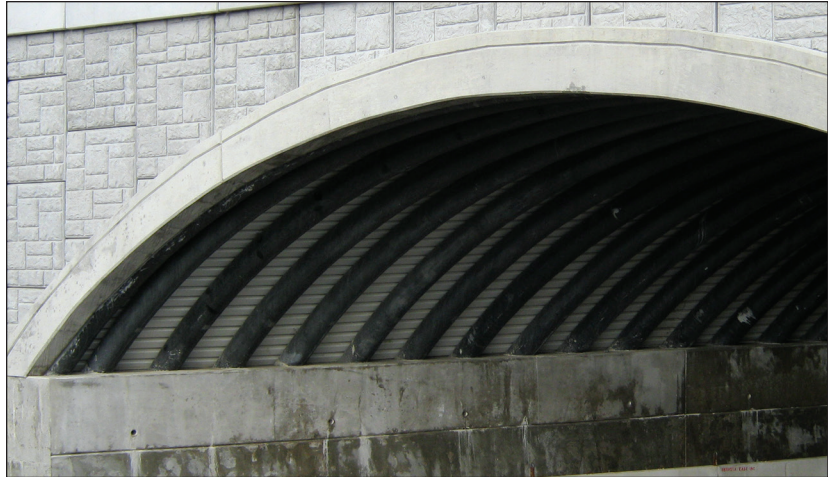
This rigidified fiber reinforced polymer arch in Caribou, Maine, which at the time of construction was the largest composite arch bridge in the world, was constructed to allow traffic to pass under a busy highway.
