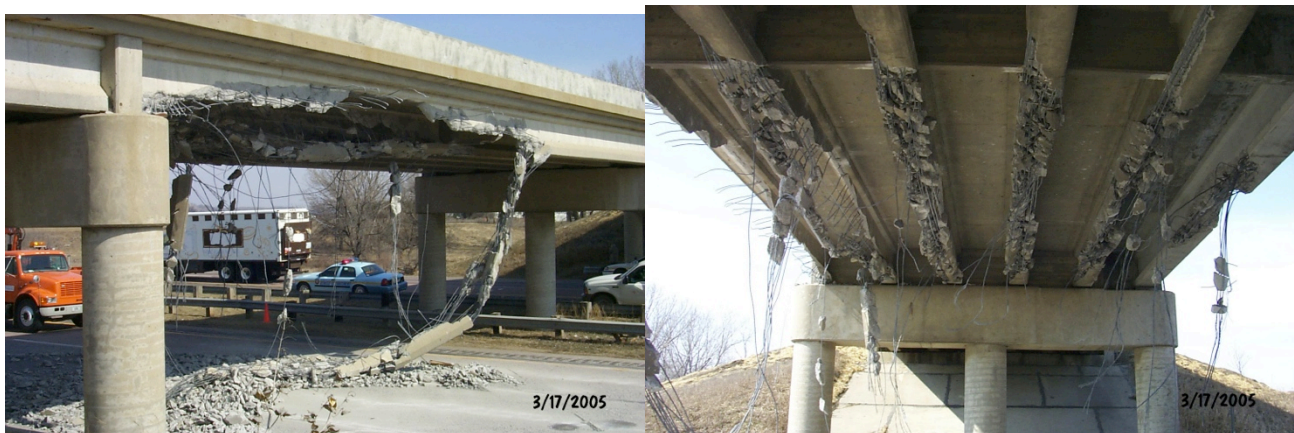
Figure 3.1 Photos Showing Prestressed Beam Bridge Impacted by Over-Height Vehicle
