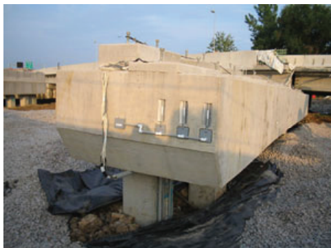
An instrumented concrete pile and cap at the Woodrow Wilson Bridge outside of Washington, DC. The instrumentation system is collecting strain and acceleration data
