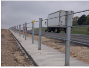
Gibraltar Cable Barrier
