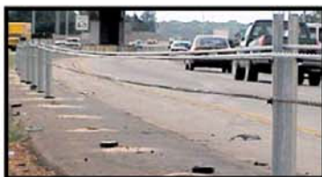
High Tensioned Rope System
