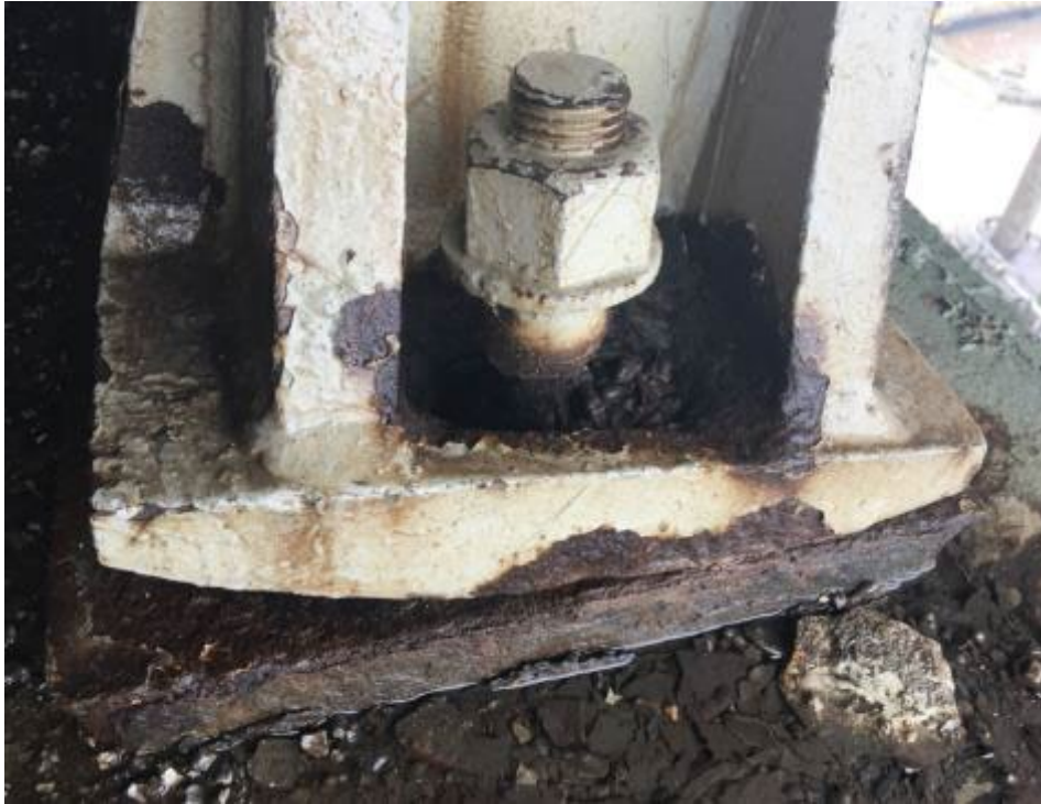
Corrosion of Steel Plates and Bolts
