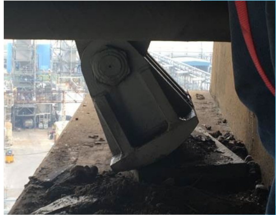
Large Rocker Rotation. Base Plate Movement. Anchor Bolt Shear-off.
