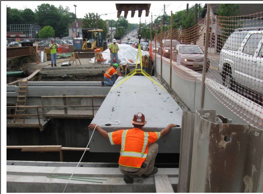
Fig 3. June 2009 - Route 23 Bridge in Cedar Grove, NJ. Ritacco Construction sets 31-foot x 6-foot HCB using excavator.
