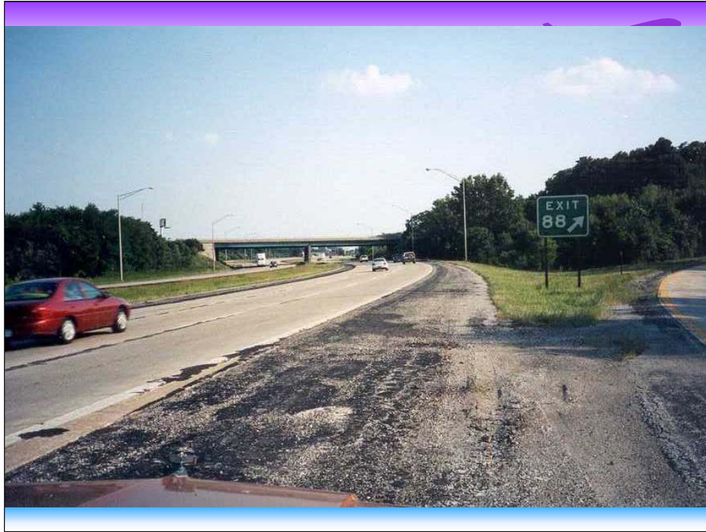
Centerline deterioration in Illinois on I-55 northbound, just south of Springfield, July 2000. The pavement is about 20 years old.
