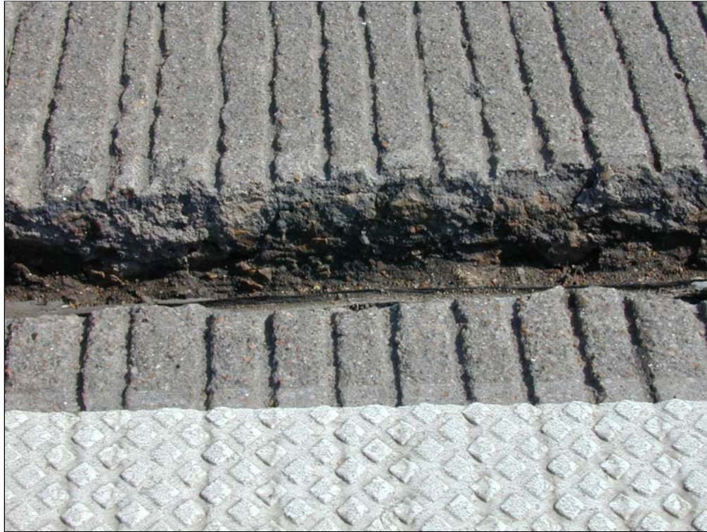
The spalled centerline joint showing failure in the paste. No broken aggregate is showing
