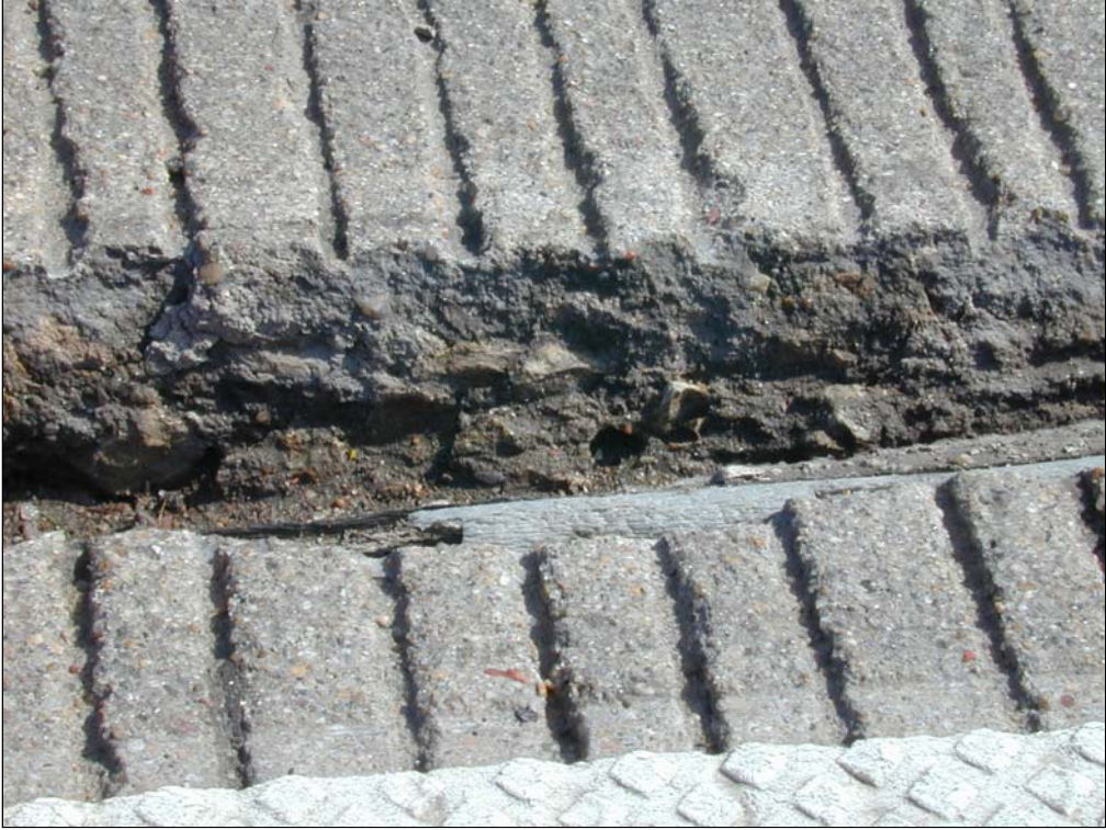
A slightly closer view of the centerline spall
