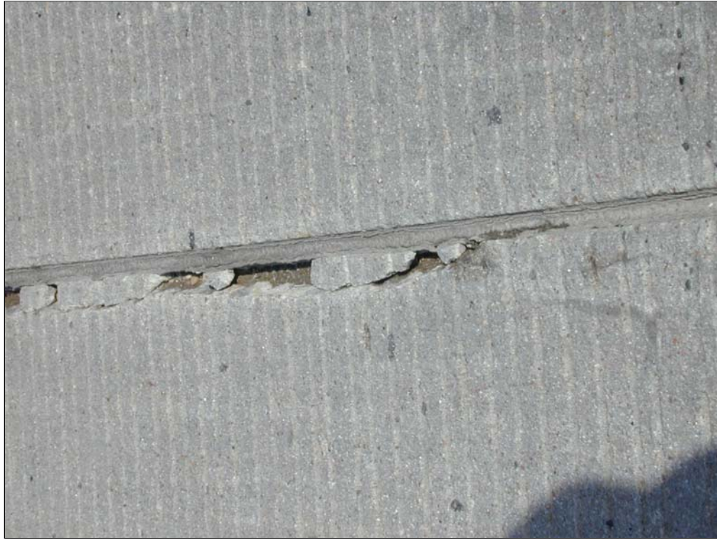
The beginning of spalling at the centerline
